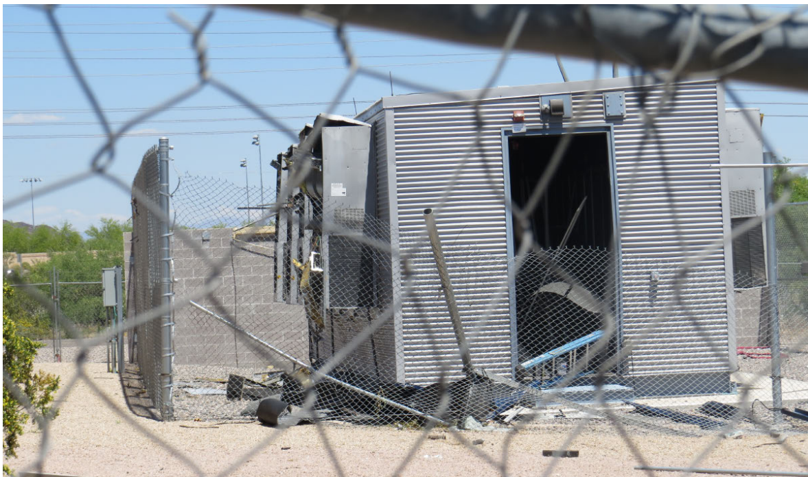
Figure 8 Additional view of debris and damage to the rear door, HVAC systems, and the container
