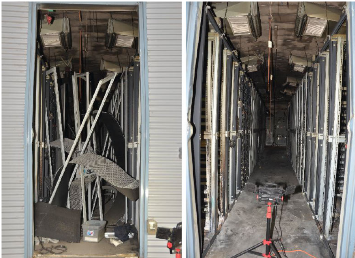
Figure 9 Interior damage to the energy storage system with the condition after the explosion (left), and condition after debris was removed to gain access to the interior and begin the forensics analysis (right)
