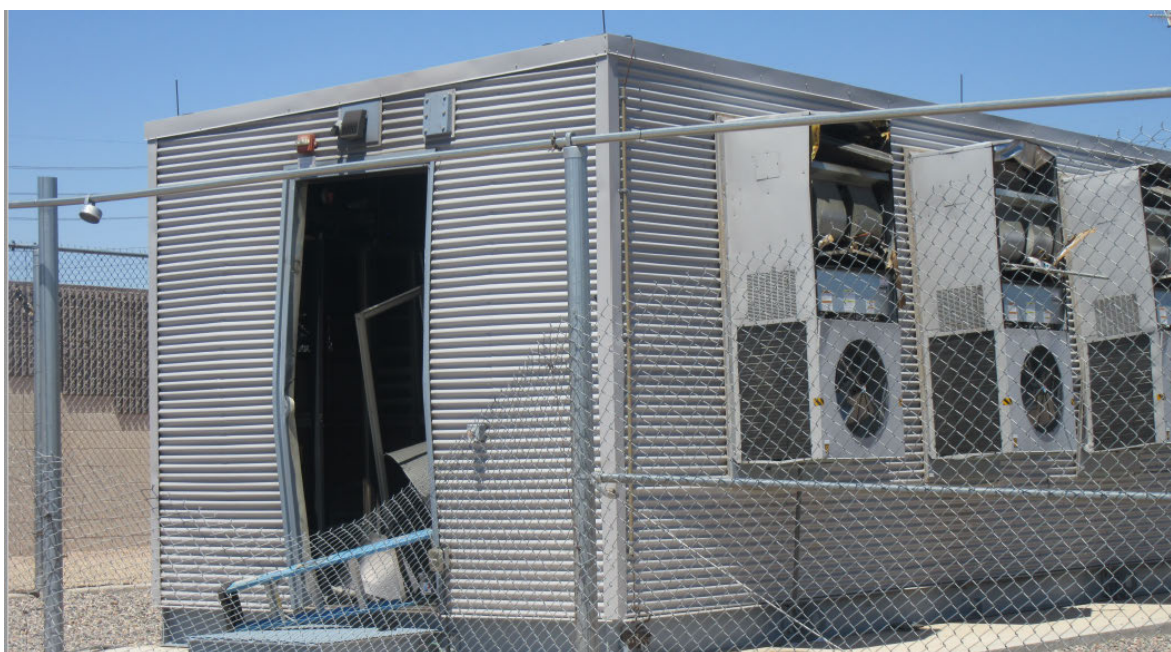
Figure 6 Damage to the rear door and HVAC systems of the McMicken BESS
