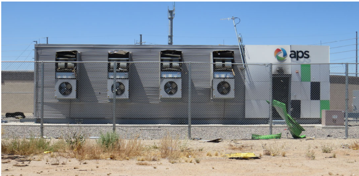
Figure 7 The side door to the McMicken BESS was ejected in the explosion and can be seen laying against the fence in the foreground
