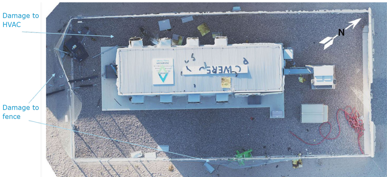
Figure 5 Aerial view of damaged BESS (image credit: Colwell Consulting)
